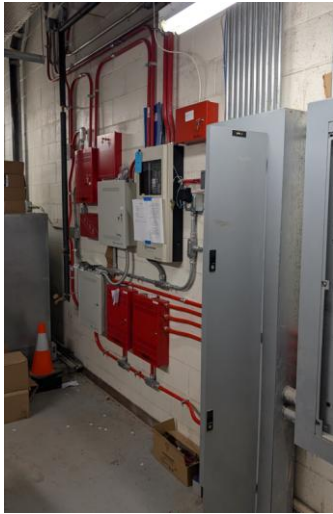
2026.08.04 – Mechanical Room 163 Fire Alarm Control Panel
